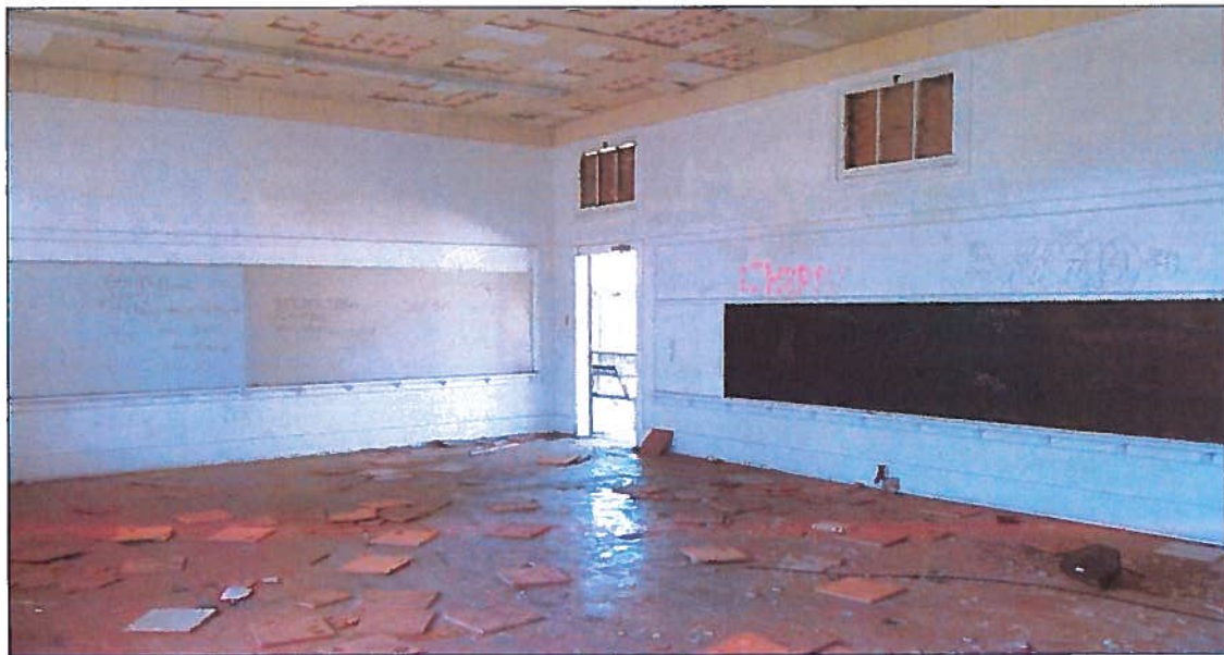
Figure 22: Classroom Detail. Classroom with wood floors, acoustic ceiling, and clerestory windows (March 18, 2016).
