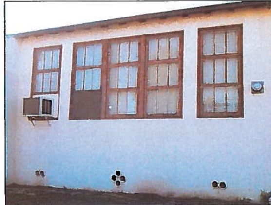
Figure 18: East Elevation Detail. Detail of east elevation wood-framed windows, canale vents, and eave (February 9, 2016).
