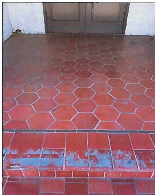
Figure 16: Tile Detail at Entrance. Detail of terra cotta tile at the primary entrance (February 9, 2016).
