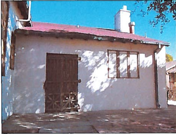
Figure 11: West Elevation View to the East. Southern portion of west elevation, view to the east. Note the chimney (February 9, 2016).
