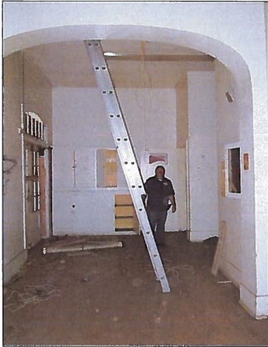
Figure 23: Arched Hallway from Main Entrance. Arched hallway, view west from main entrance (March 18, 2016).
