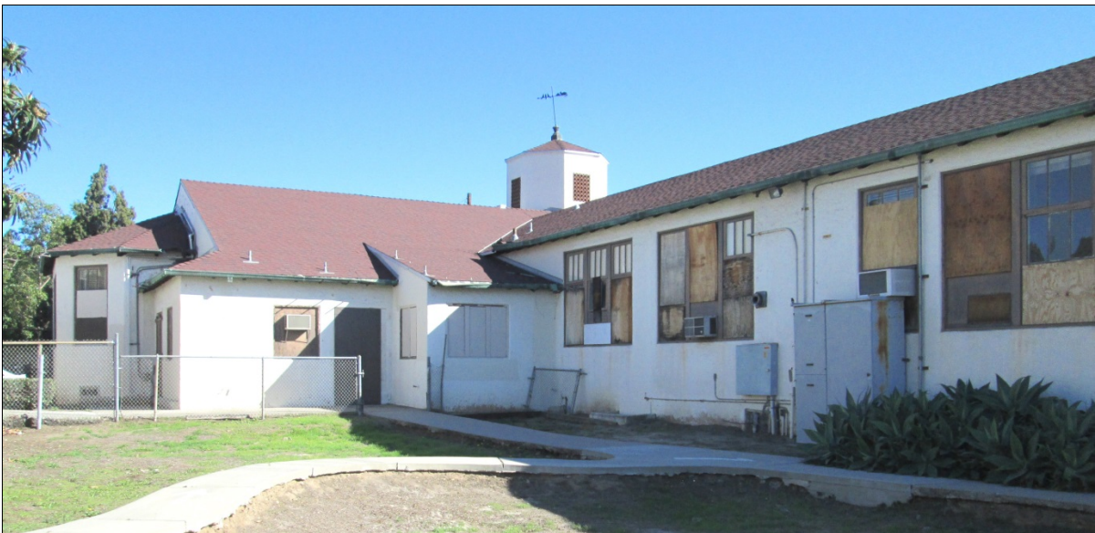
Figure 6: North Elevation. North elevation, view to the east. Note bay window on left side of photograph.
