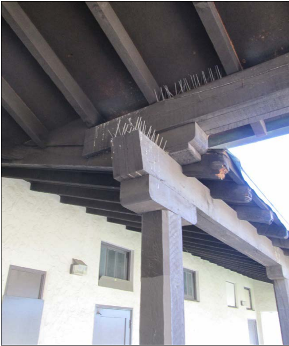
Figure 7: Posts and Rafters Detail. Detail of chamfered posts, bull nosed brackets, and exposed rafters (February 9, 2016).
