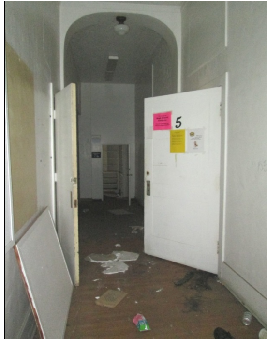
Figure 24: Arched Hallway from Secondary Entrance. Arched hallway, view west from secondary entrance (March 18, 2016).
