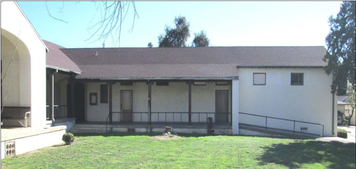
Figure 5: South Wing of West Side. South wing of west side of school, view to the south (February 9, 2016).
