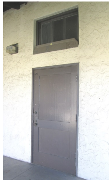
Figure 10: Wood Door and Clerestory Window Detail. Detail of wood door and clerestory window in west elevation (February 9, 2016).
