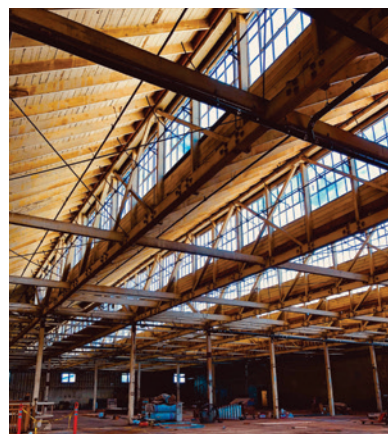
CHAPMAN'S VILLA PARK ORCHARD PACKING HOUSE Historic restoration includes 350 multi-pane windows restored by the Spectra Company, and more than 100 tons of steel to seismically strengthen the structure to last another 100 years.
